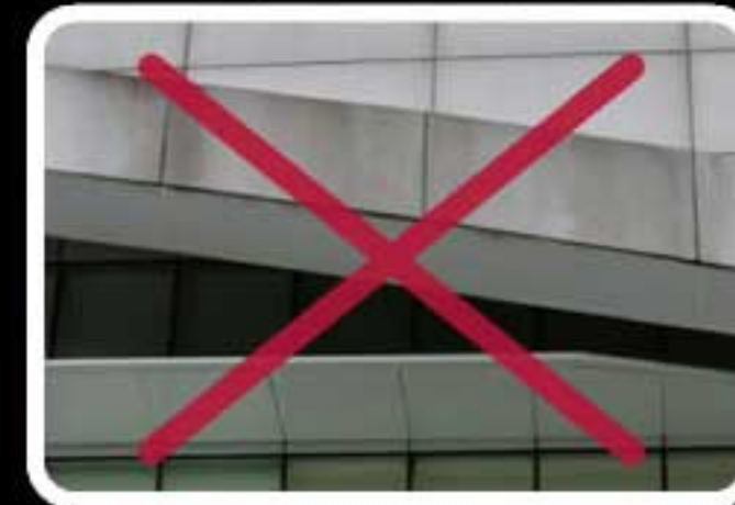
Streaking (Silicone Sealant)
