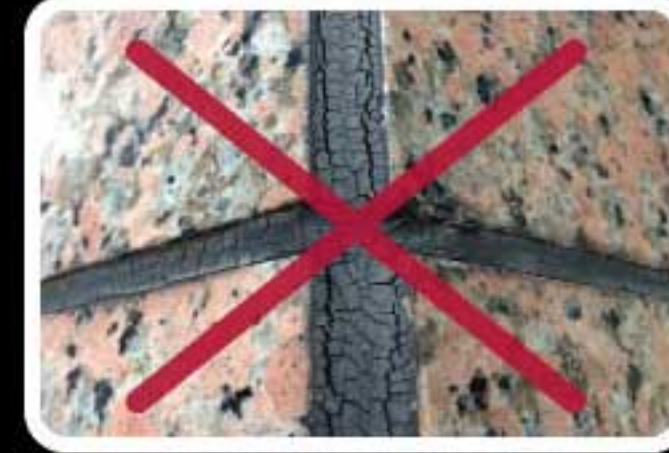
Poor UV resistance - Sealant cracking (PU Sealant)
